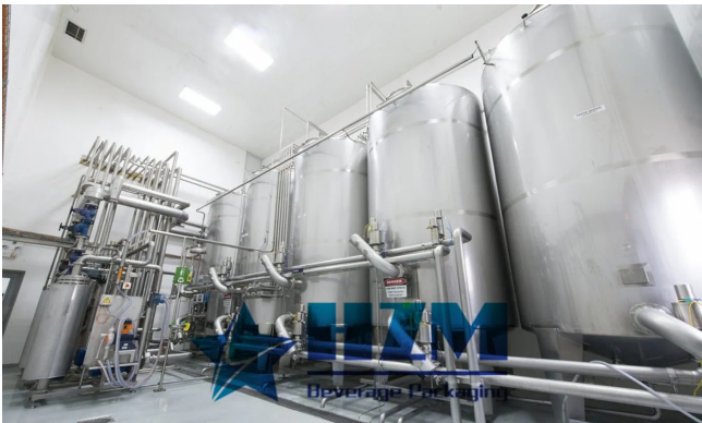
Figure 2. Beverage processing tanks and sanitary pipework from the HZM equipment library. This photograph illustrates the processing area, not a complete line layout.
